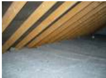
Example loft insulation
